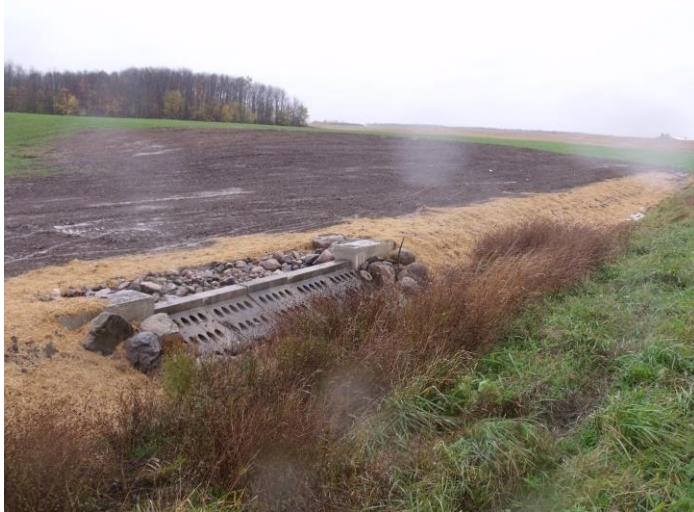
Installation of an earthen berm with drain and grassed waterway. Credit: Pine River Watershed Initiative Network.
